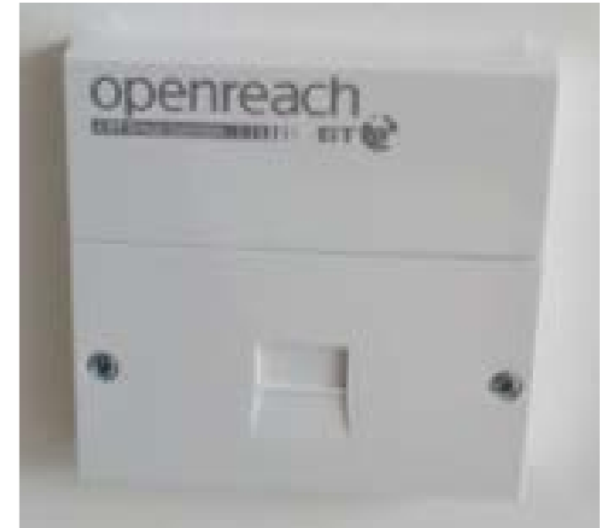
BT phone socket adjacent to double electric socket in hall cupboard
