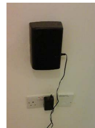
Satellite/TV amp located in hall cupboard
